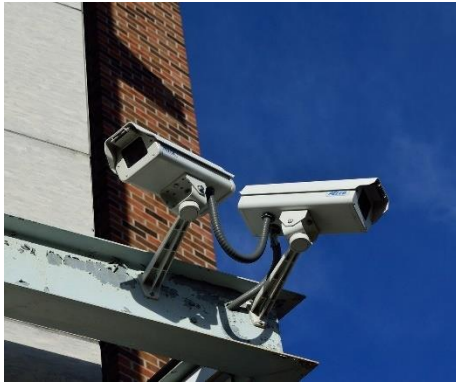
Figure 3: CCTV can be highly visible and will contribute to both deterring and detecting an adversary.
