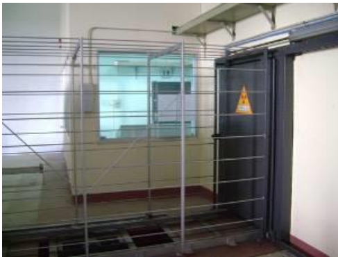
Figure 7: Security door and fencing (Courtesy of Gamma-Service Recycling GmbH)
