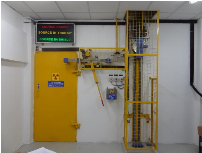
Figure 9: Access to the irradiator cell should be via a hardened security door fitted with opening detection sensors. Security can work hand in hand with safety, for example by interlocking a mechanical latch bar with the mechanism for lowering the source rack into a safe position as shown. The security of this mechanism, including encasement and tamper detection, should be considered. Illustration courtesy of Symec Engineers.
