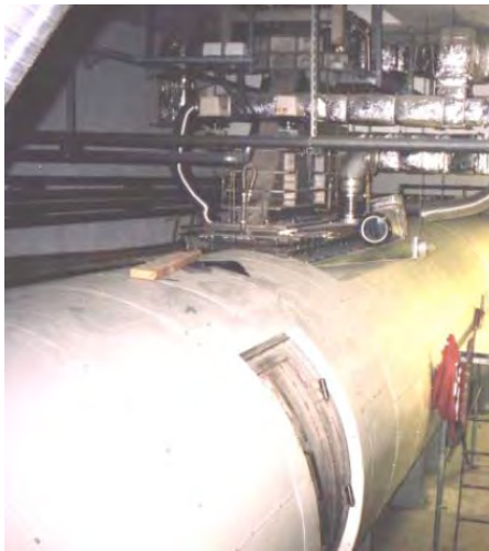
Figure 113. Flue Gas Irradiation Chamber with EB Unit
